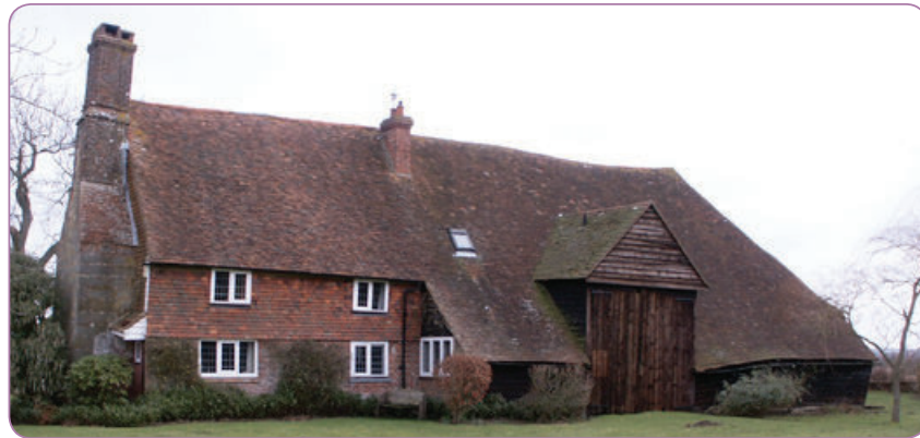
ABOVE A linear farmstead, with the house and working buildings attached in one range, is very unusual in Kent. (© Bob Edwards)
